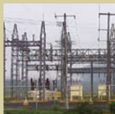
ELECTRIC SUBSTATION STRUCTURES
