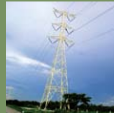
SUBTRANSMISSION AND TRANSMISSION TOWERS
